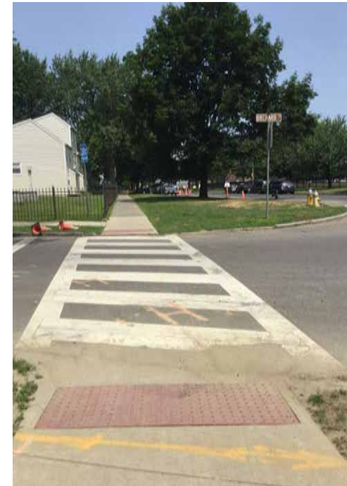
Along Plainfield Street, new ladder crosswalks with curb ramps have been installed.
