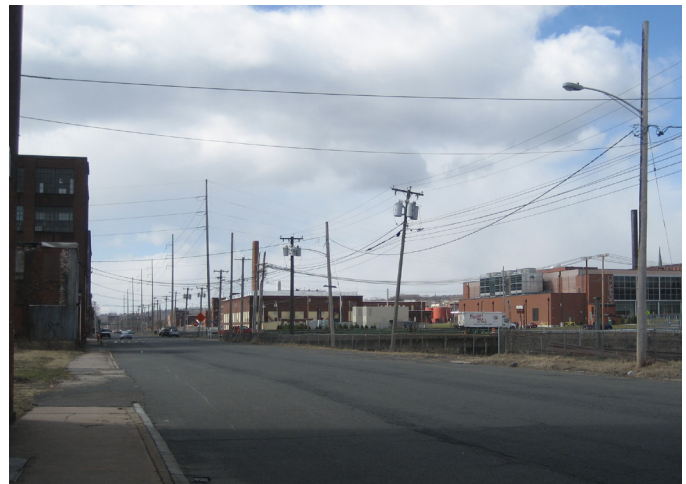
Race Street has few pavement markings and sidewalks in need of repair.
