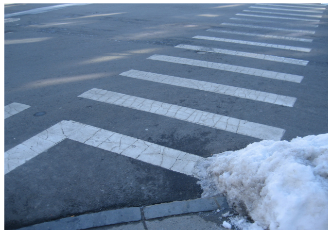
The painted crosswalks throughout the study area use the continental painting pattern.
