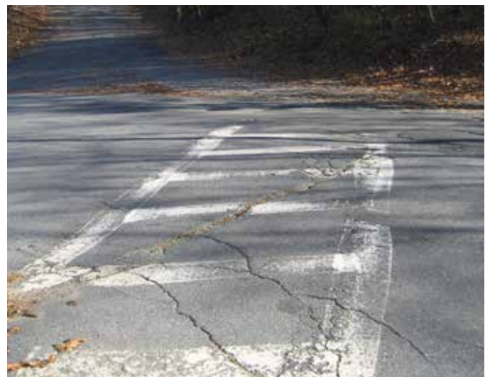
The crosswalk at the Baker and Harvard Street intersection needs to be either removed or repainted.
