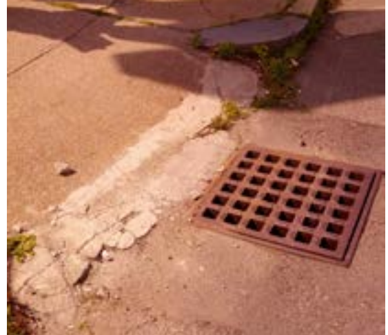
Broken curb ramp and storm drain
