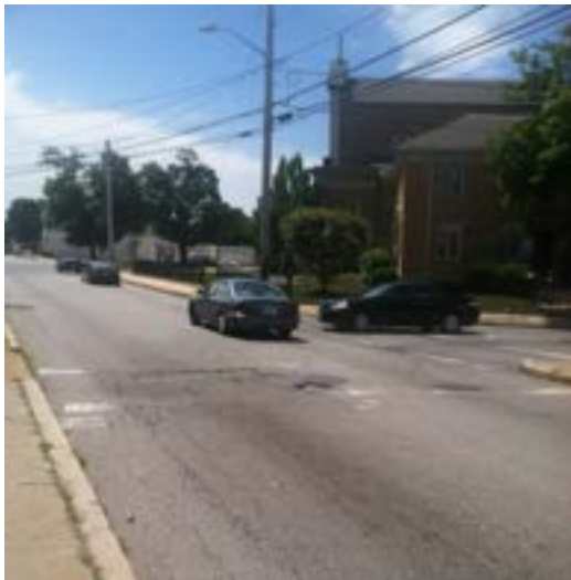
Faded crosswalk at proposed three-way stop at Stafford and Tucker Streets
