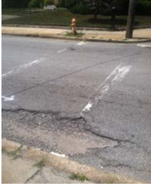
Faded crosswalk with pothole at Stafford and Tucket Streets
