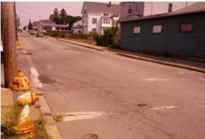
Faded crosswalk at bus stop on Stafford Street
