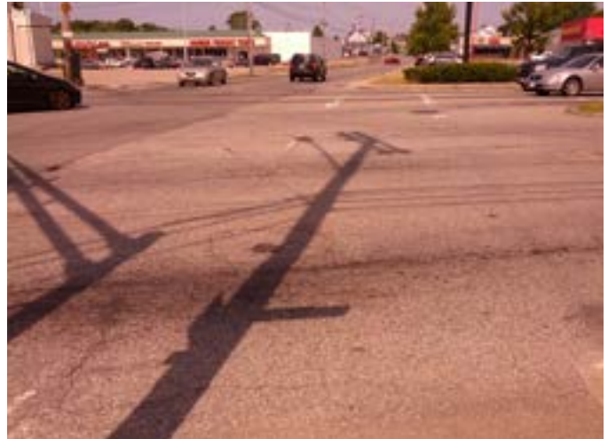
Faded crosswalk at Canning Boulevard
