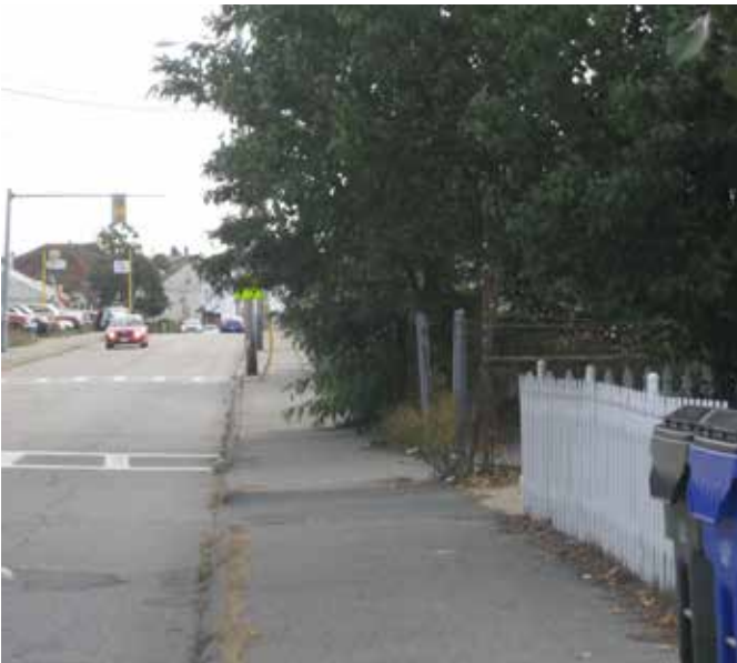
Vegetation overgrowth on Pine Street
