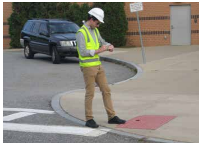
Peeling detectable warning strip near the elementary school
