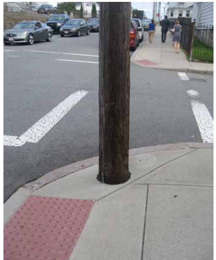
Telephone pole blocking curb ramp across Pine Street
