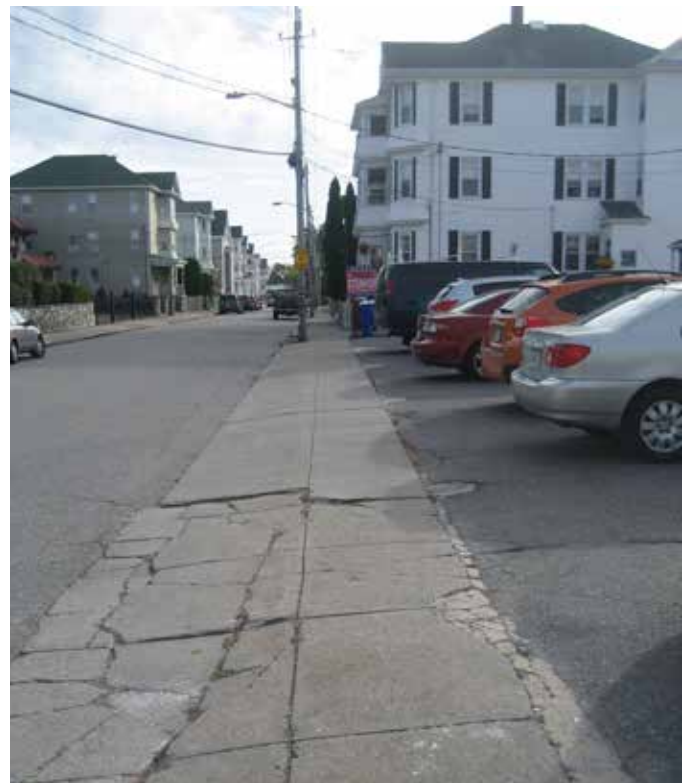
Broken sidewalk and extensive curb cut on Bedford Street
