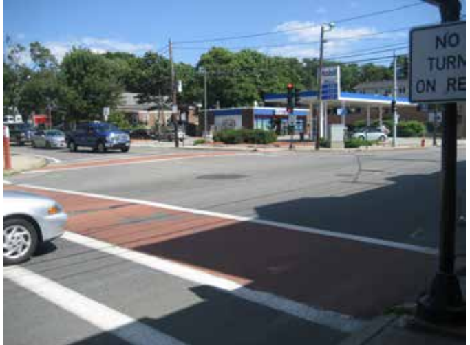
Crosswalks at the Main Street/Greenwood Street/Oak Street intersection need to be resurfaced.
