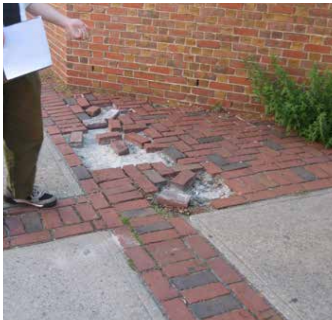
Loose bricks along Washington Street
