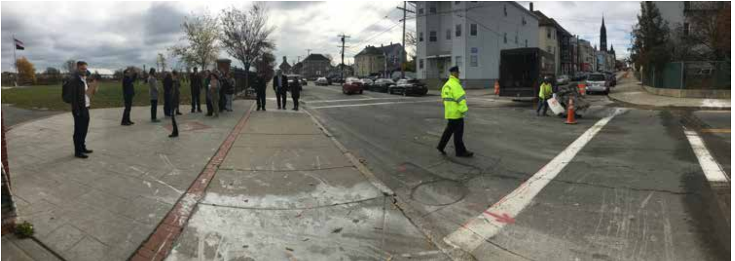
Wide angle view of the Belleville Avenue/Bullard Street intersection and the future site of a public art mural on the roadway. Curb ramp construction was underway during the walk assessment.
