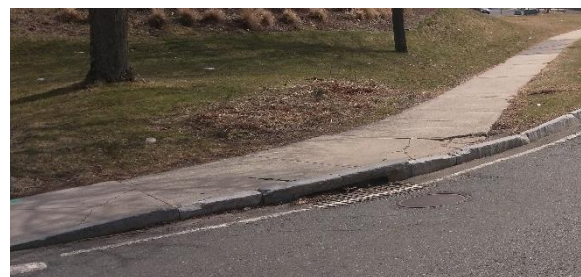
Image 3: Sidewalk deterioration along right-turn slip lane on Resnic Boulevard northbound approach.
